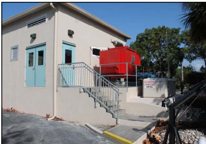
New Diesel Back-Up Pump
