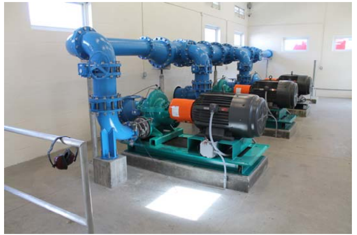
Three 150 HP, 2,500 GPM electric pumps
