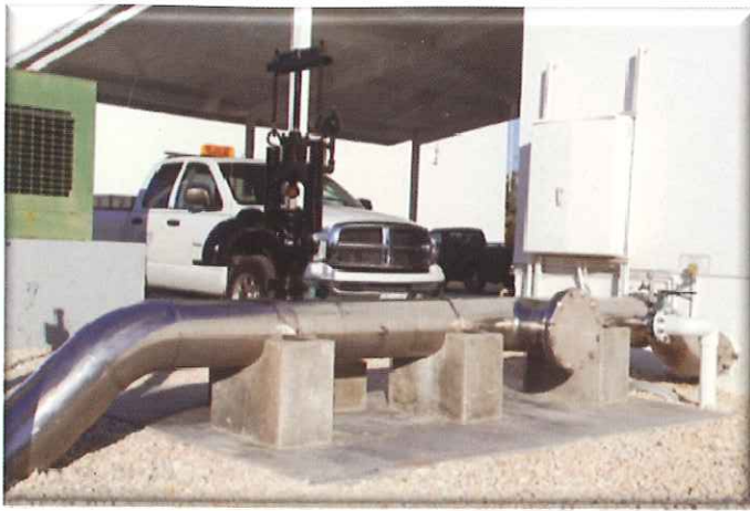
Stainless Well Line Header
