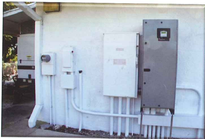
Main Office Transfer Switch
