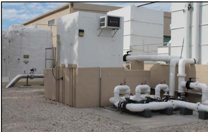
Current Brine Clearwell with Three Centrifugal Pumps sitting at Ground Level
