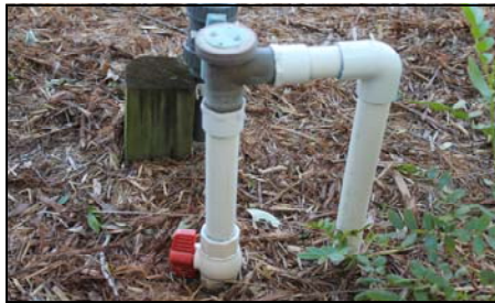
Irrigation System Vacuum Breaker
