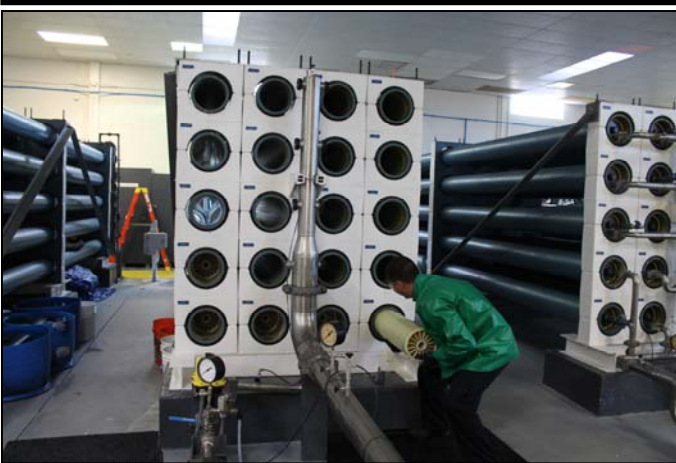
E Train Membrane Removal
