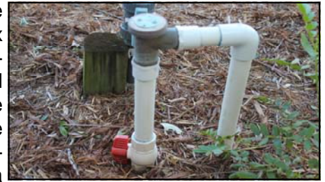
Irrigation System Vacuum Breaker
