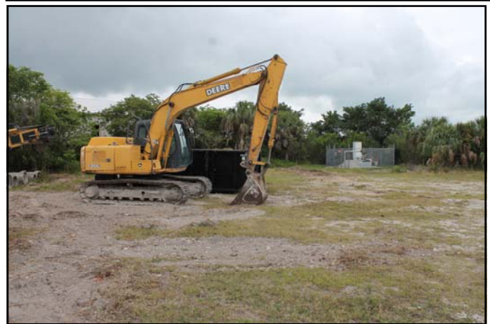
Site Prep Work at New Suwannee Well Site (S9) H13 is Behind the Small Fence in the Background
