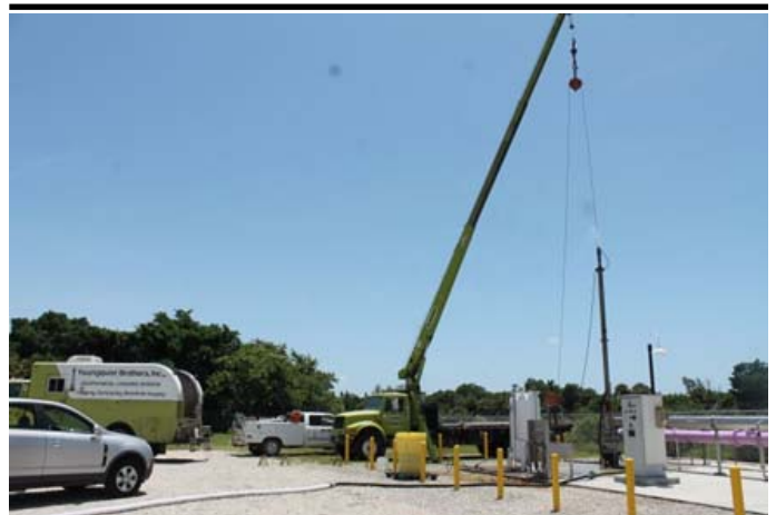
Crane with Bore Camera for Visual Inspection of the 3200' Deep Well as Part of our Injection Well 5 Year MIT
