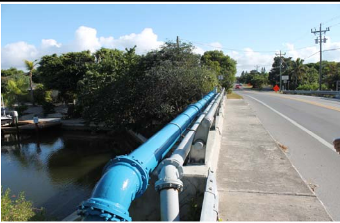
8" Ductile Iron pipe across the East Periwinkle Way bridge
