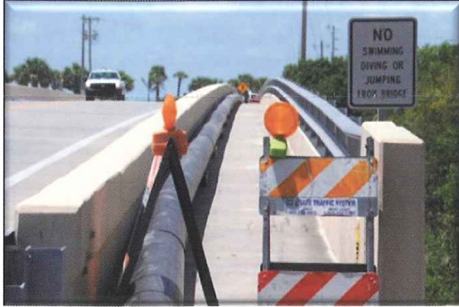
Temporary 12" HDPE pipe that will supply water to Captiva while the old main is removed and replaced.
