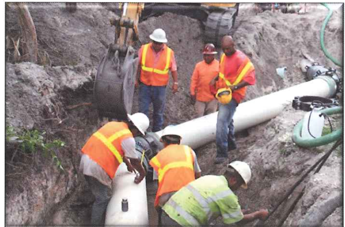
Contractor Ken Cabana overseeing the connection between the new well line and the existing line
