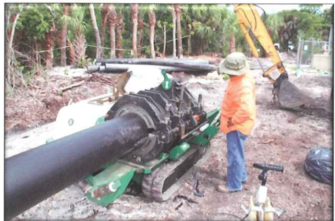
Welding a flange adaptor to the 12" HDPE bore pipe that was "pulled" under Sanibel-Captiva Road
