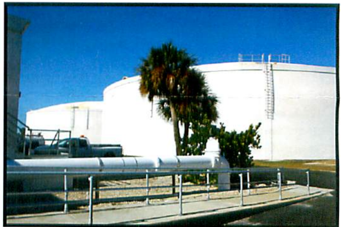
Twin five million gallon storage tanks located at the RO Plant
